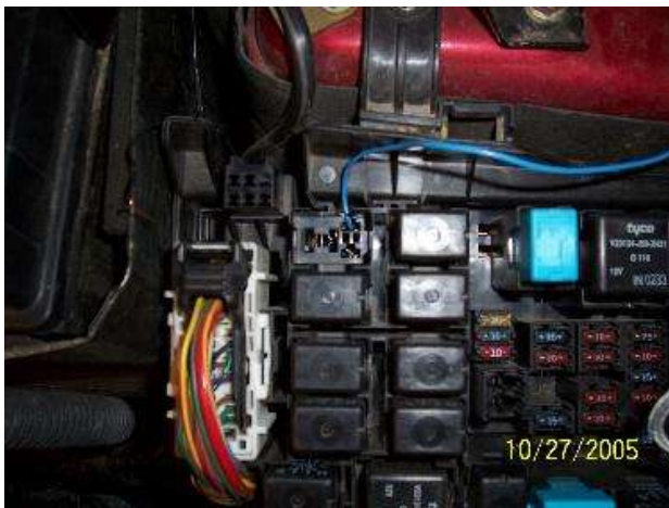
Connect the Blue Fan Relay wire here.
