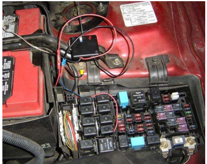
Connect the power and fan control leads.
